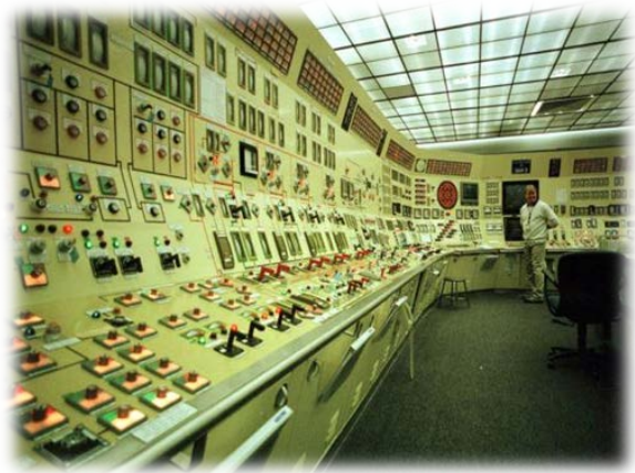
Figure 18. Typical nuclear power plant control room with analog technology.
