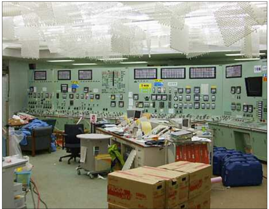
The Unit 1 control room on March 24, after lighting was restored. (Photo: Tokyo Electric Power Company/Kyodo via AP Images)
