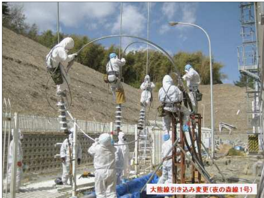
On March 18, workers repair equipment in an effort to restore off-site power to Units 3 and 4 at Fukushima Daiichi. (Photo: Tokyo Electric Power Company/Kyodo via AP Images)
